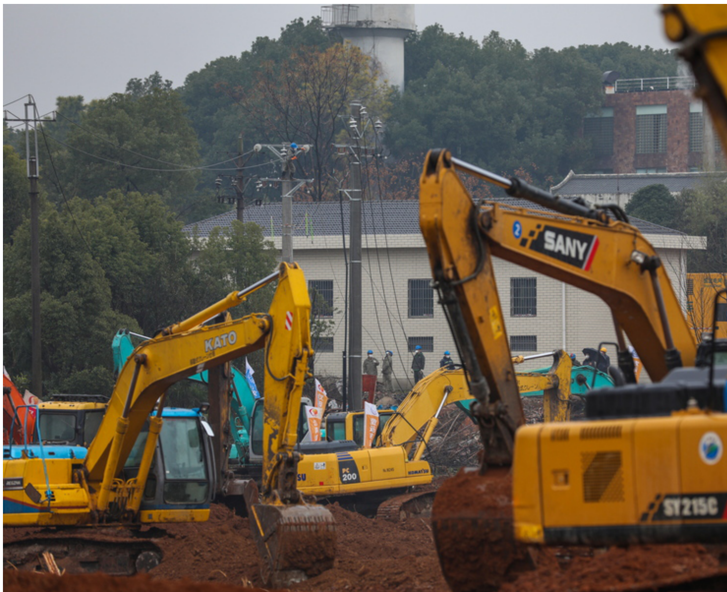
epa08157639 People work at the construction site of a field hospital in Wuhan, Hubei province, China, 24 January 2020. The hospital is expected to be completed by 03 February 2020 to cope with the increasing number of people affected by the coronavirus. The coronavirus has so far claimed 25 lives and infected more than 800 others, according to media reports. The virus has spread to Thailand, South Korea, Japan, Singapore and Taiwan. EPA/YUAN ZHENG CHINA OUT
