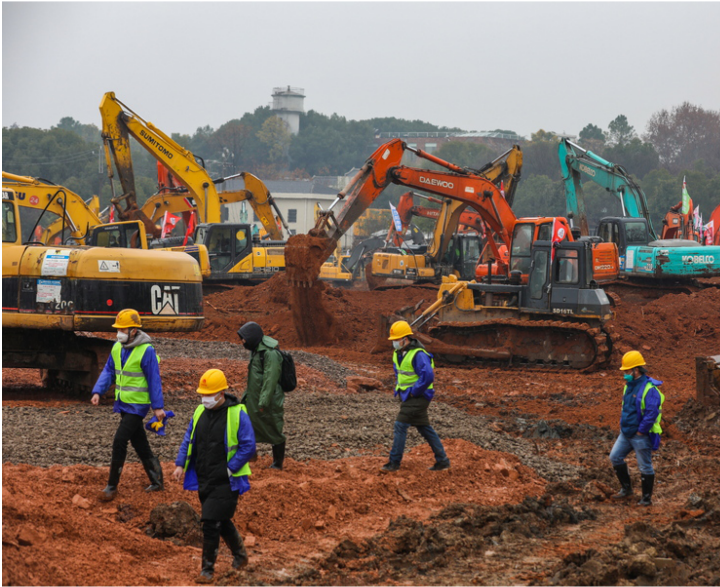
epa08157643 People work at the construction site of a field hospital in Wuhan, Hubei province, China, 24 January 2020. The hospital is expected to be completed by 03 February 2020 to cope with the increasing number of people affected by the coronavirus. The coronavirus has so far claimed 25 lives and infected more than 800 others, according to media reports. The virus has spread to Thailand, South Korea, Japan, Singapore and Taiwan. EPA/YUAN ZHENG CHINA OUT
