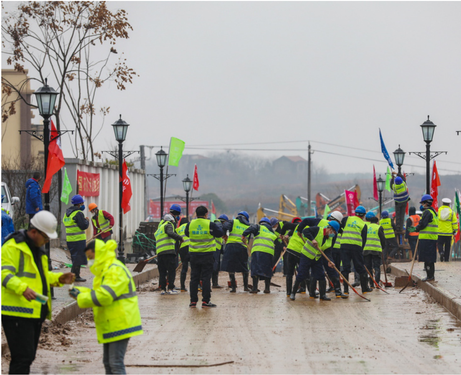
epa08157640 People work at the construction site of a field hospital in Wuhan, Hubei province, China, 24 January 2020. The hospital is expected to be completed by 03 February 2020 to cope with the increasing number of people affected by the coronavirus. The coronavirus has so far claimed 25 lives and infected more than 800 others, according to media reports. The virus has spread to Thailand, South Korea, Japan, Singapore and Taiwan. EPA/YUAN ZHENG CHINA OUT
