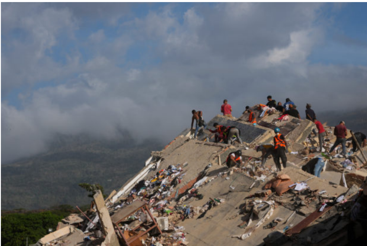
Rescue workers search through the rubble of a building that collapsed when earthquakes struck Catia La Mar, Venezuela, Monday, June 29, 2026. (AP Photo/Matias Delacroix)
